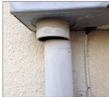
Earth movement resulting in PVC raceway being pulled loose from the male adapter
